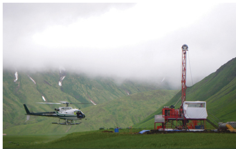
Helicopter-supported geothermal exploration drilling on Akutan Island, Alaska. Photo credit: Neil McMahon
